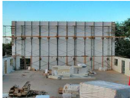
Three Story Insulating Concrete Forms Wall Construction, Note the Stacked Styrofoam Form Panels
