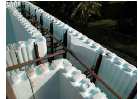
Insulating Concrete Forms Wall Construction Details Showing Styrofoam Form Panels, Steel Spacers and Rebar
