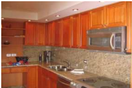
Complete Kitchen Remodel including New Cabinets, Granite Counters, Flooring, Plumbing, Electrical, Sliding Doors and Windows, Wahiawa, Hawaii
