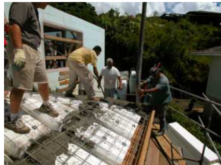
Insulating Concrete Forms Construction, Three Story Home with ICF Walls, Floors and Hip Roofs, Makiki Heights, Honolulu, Hawaii
